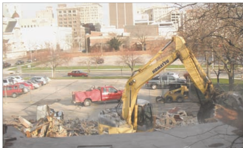
Demolition of the Lawyer's building on Dec. 8, 2011 could result in additional parking for Sinclair.
